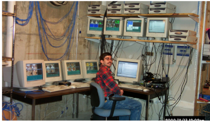
Figure 1.1: Smart Environment Server Room (Source: Aware Home project, Georgia Tech)
