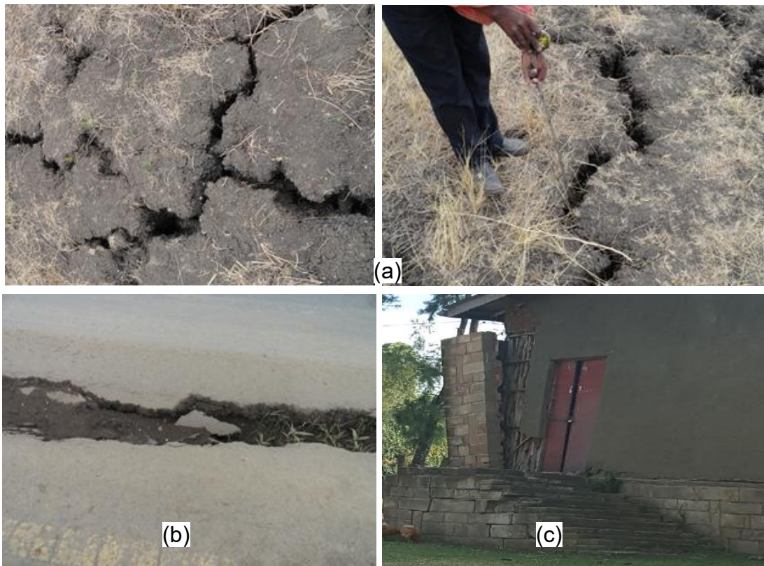
Figure 1.1: Typical BC soil damages in Ambo, Ethiopia: a) BC soil cracks during dry season, b) typical crack scene on roads and c) a serious damage on a house constructed on BC soil
