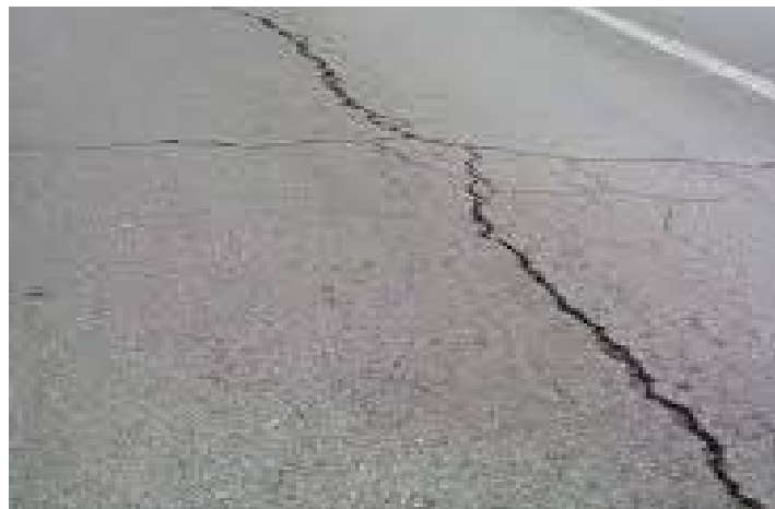
Figure 2.14: Typical longitudinal crack developed on pavements over expansive clays (After [75])
