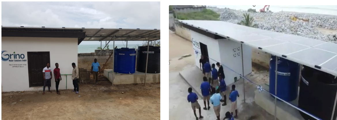
Figure 44 the pilot project was installed in October 2020, and performance data were gathered using a remote monitoring system. 8 kWp panels were installed to power the system.
